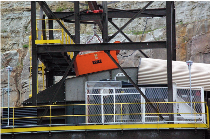
Figure 1. Suspended magnet: the magnet is suspended over the conveyor belt to remove ferrous tramp from the coal before crushing. In this application the magnet is suspended over the material discharging the head pulley.
